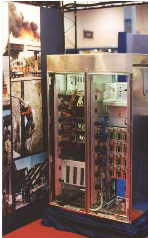
A 2001 ITS Annual Meeting main attraction, the Advanced Traffic Management System (ATMS) that is being deployed throughout the greater Houston metropolitan area.
